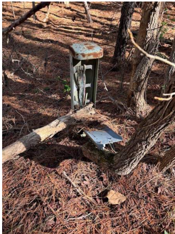
Photograph 6: View of Utility Box, open, facing southeast
