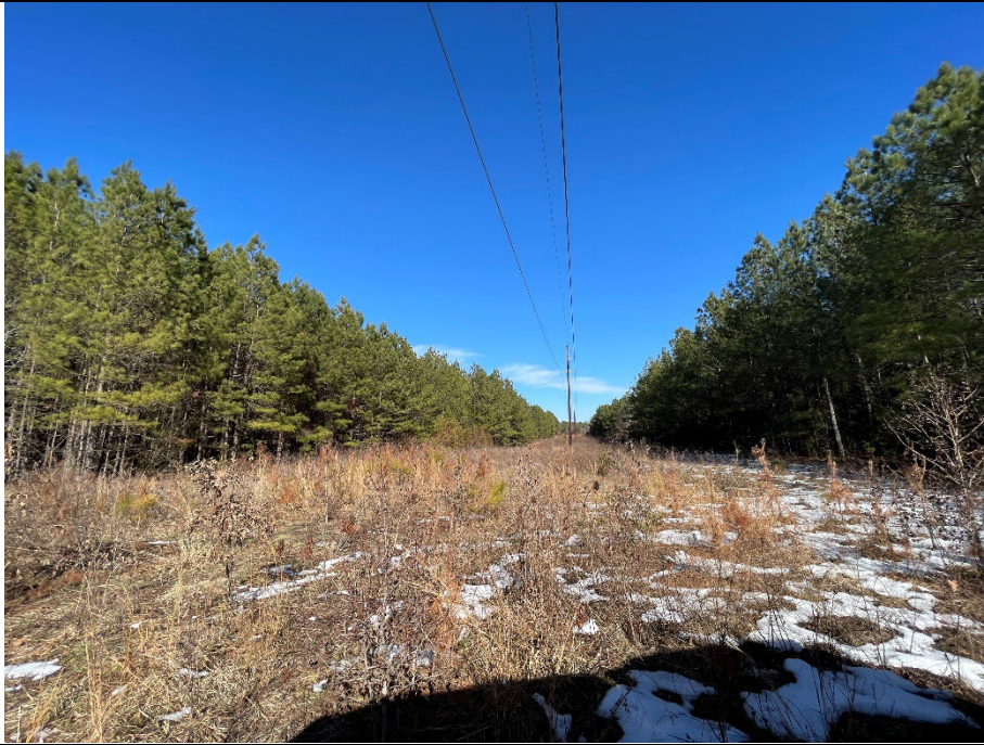
Photograph Number 21: Facing northeast at an overhead utility crossing Johnson Pond Lane within the western extent of the PSA.
