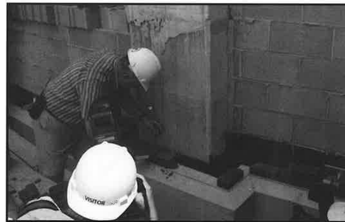
Roland Slimmer places the first of 1.2 million bricks to be used in the construction of Baltimore's new NFL stadium.
