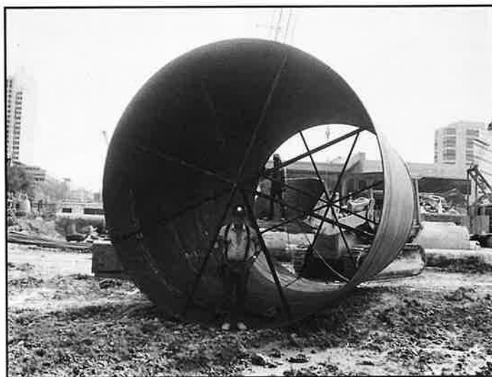
TOM PETERMAN OF THE LONG FOUNDATION COMPANY STANDS INSIDE CAISSON BEFORE INSTALLATION ON THE CONVENTION CENTER EXPANSION SITE
