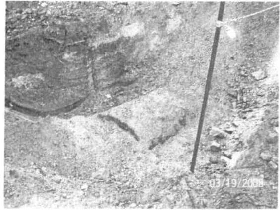
Photograph 2: Gasoline Tank Prior to Removal
