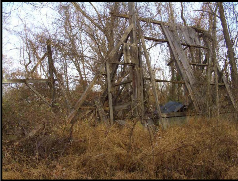
Figure 6. T. Watkins Site (18PR1028). View to the Southwest of Collapsing Barn on the Western Edge of the Site.
