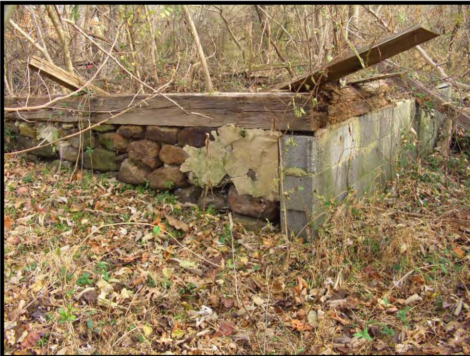
Figure 7. T. Watkins Site (18PR1028). View to the Northeast Showing Fieldstone Foundation of Outbuilding with Multiple Repairs.
